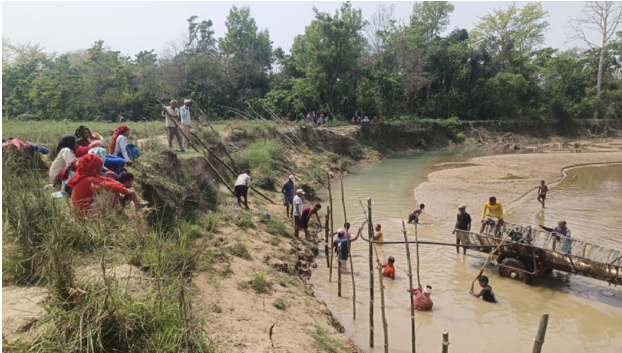
Tole members took an initiative to construct bio-embankment using local resources i.e., bamboo and sand racks at Jaljaliya, Bhajani rural municipality, Tikapur
